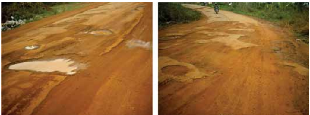
Plate 1. Failed section of Luba–Erunwon axis of Ijebu-Ode–Erunwon road
