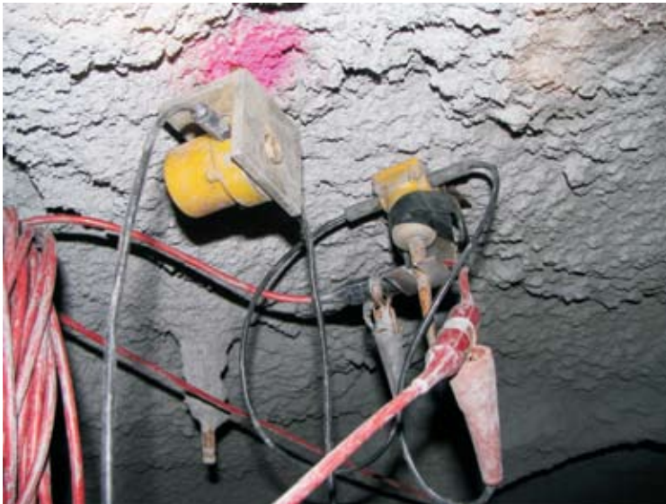
Figure 3. Vertical and horizontal geophone mounted on the ceiling of exploration gallery
