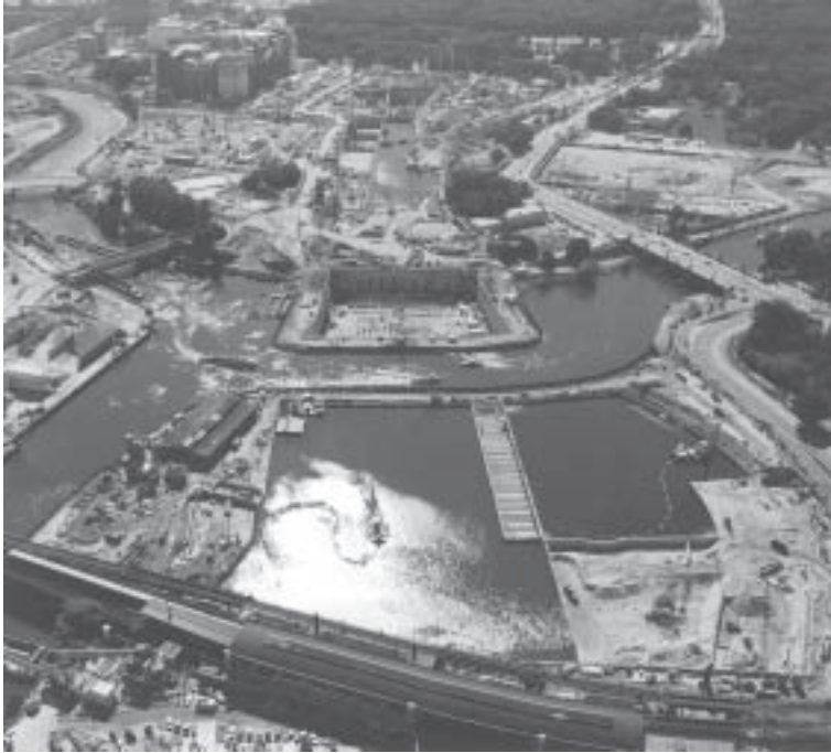
Figure 1. In front a construction pit with subaquatic concrete floor, in the back different construction levels of the troughs and in the upper area a part of the Tiergarten Park is visible.
