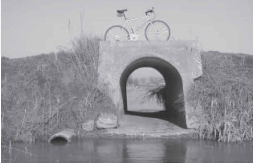
Figure 2. In situ evidence of the land subsidence that has turned a bridge into a useless structure. The left drainpipe helps convey the water of the channel originally flowing through the protruding infrastructure
